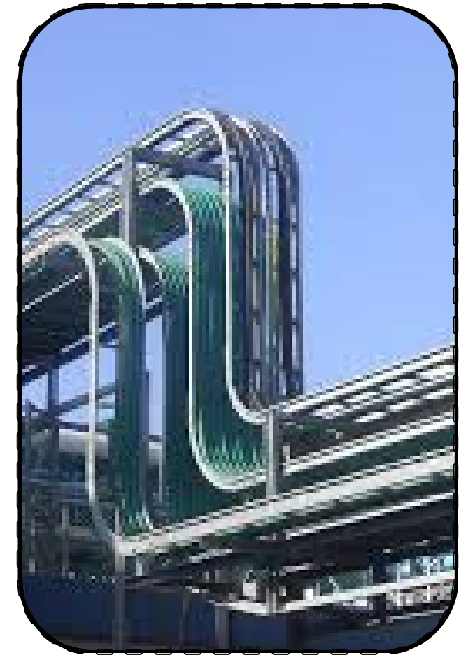
HUGE NETWORK OF CABLES
