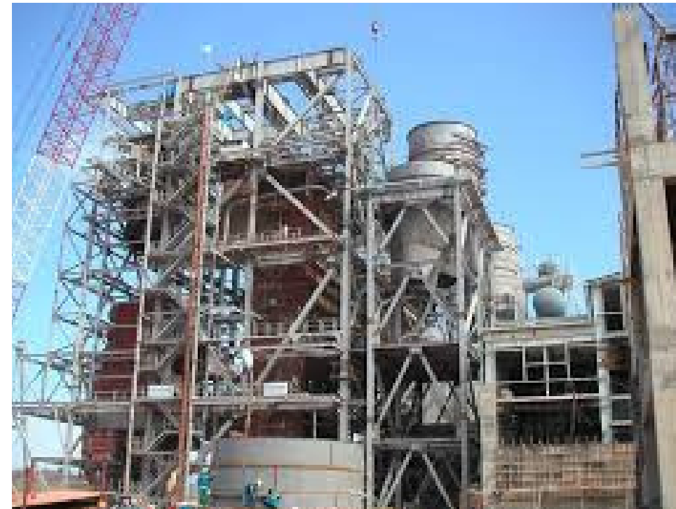
INDEPENDENT STRUCTURES TO SUPPORT DUCT , CONVEYING SYSTEMS AND CABLES
