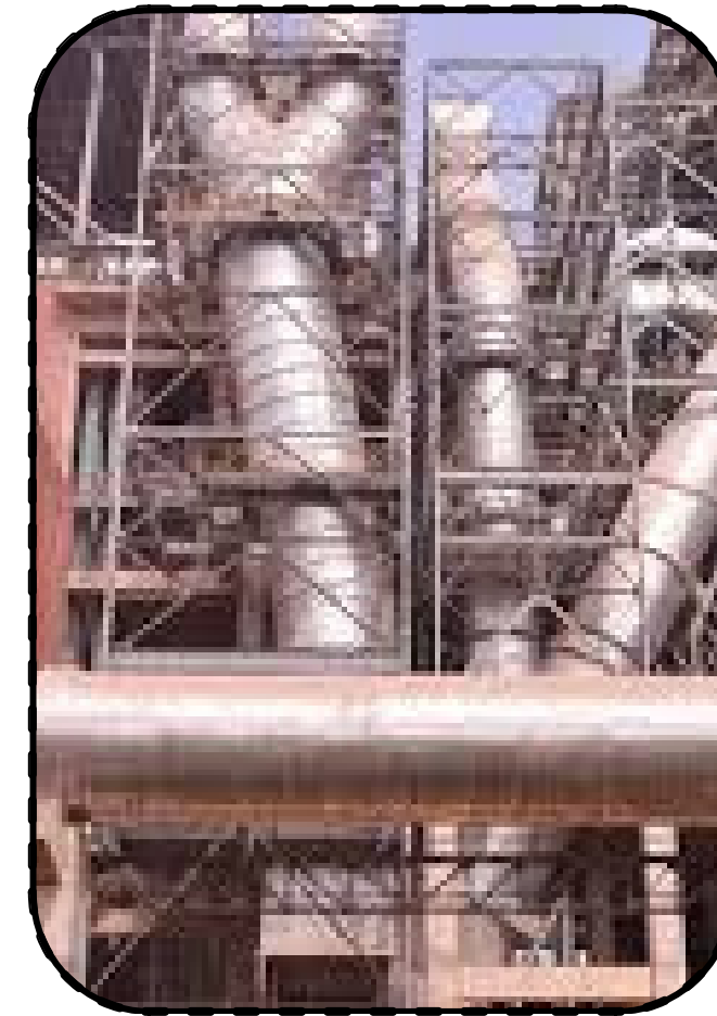
HUGE INTERCONNECTING DUCT NETWORKS
